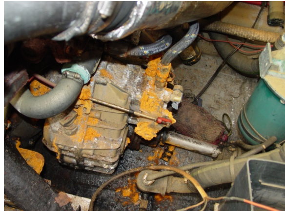
Photo 5: Example of engine corrosion
